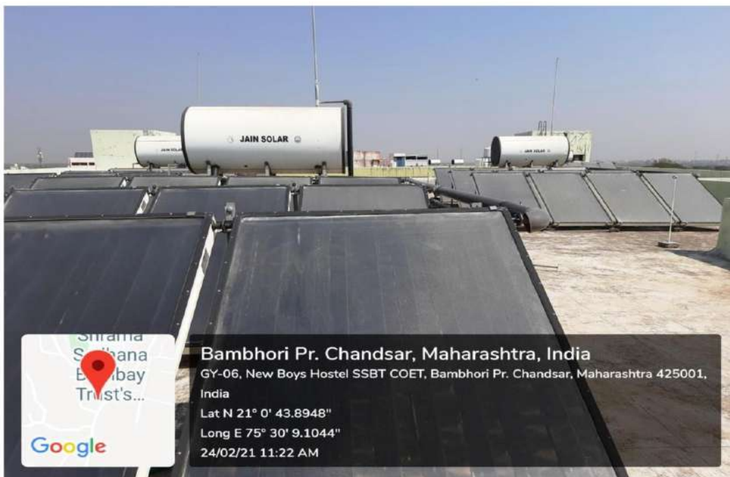
Fig . No.2 Solar Water Heater at Hostels' Rooftop
