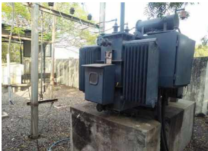
Fig No.1 11kV/433V, 500kVA OLTC Transformer
