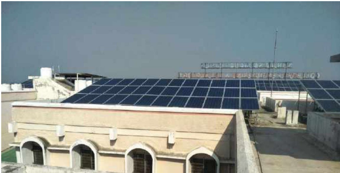
Fig No. 3 290kWp On Grid PV Solar Rooftop Power Plant
