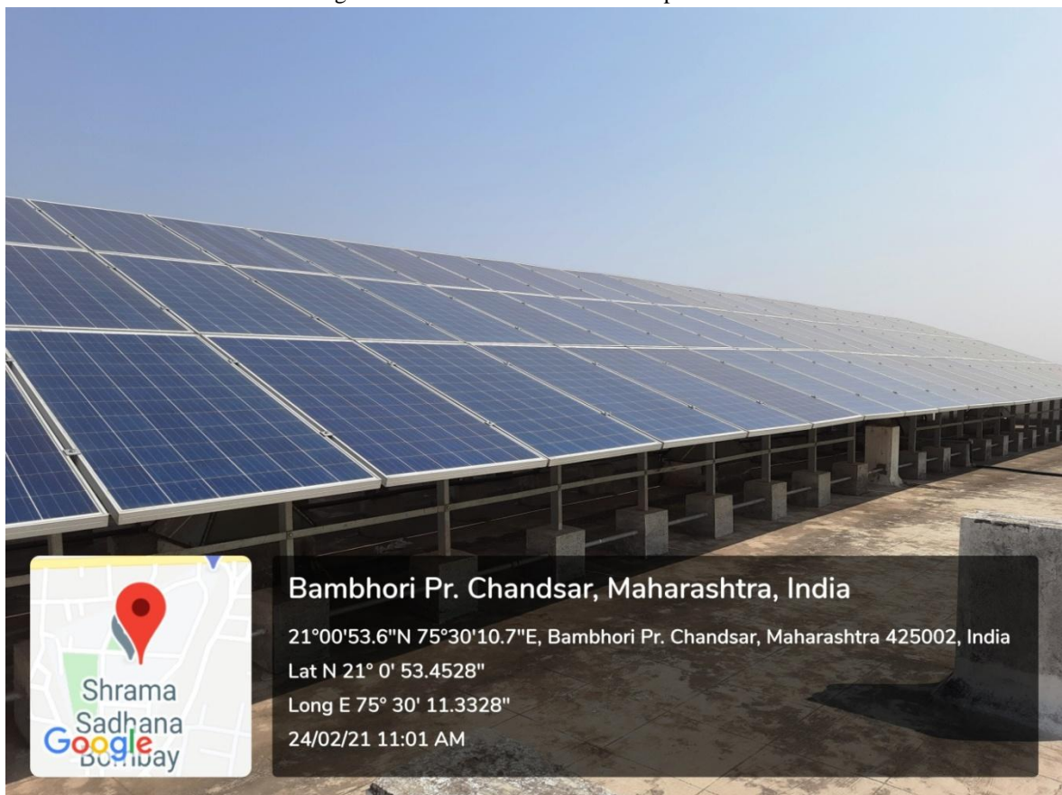
Fig. No. 3 On Grid PV Solar Rooftop Plant
