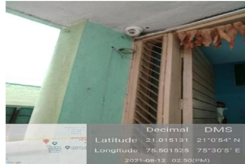
CCTV AT Girls Hostel
