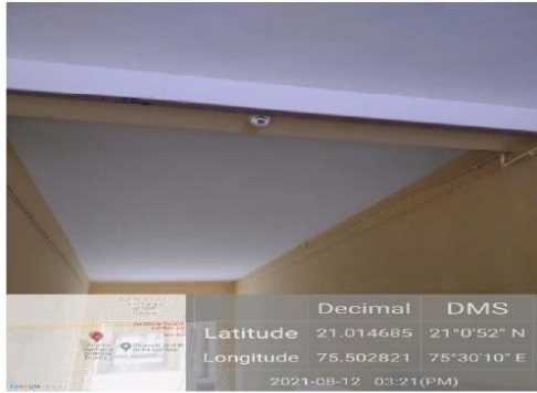
CCTV AT CORRIDOR
