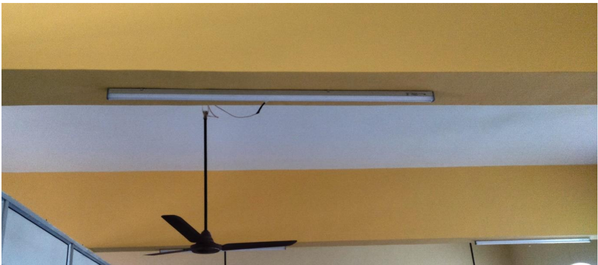
Fig. No.3 Fluorescent Tub Light replaced by LED Tube Fitting
