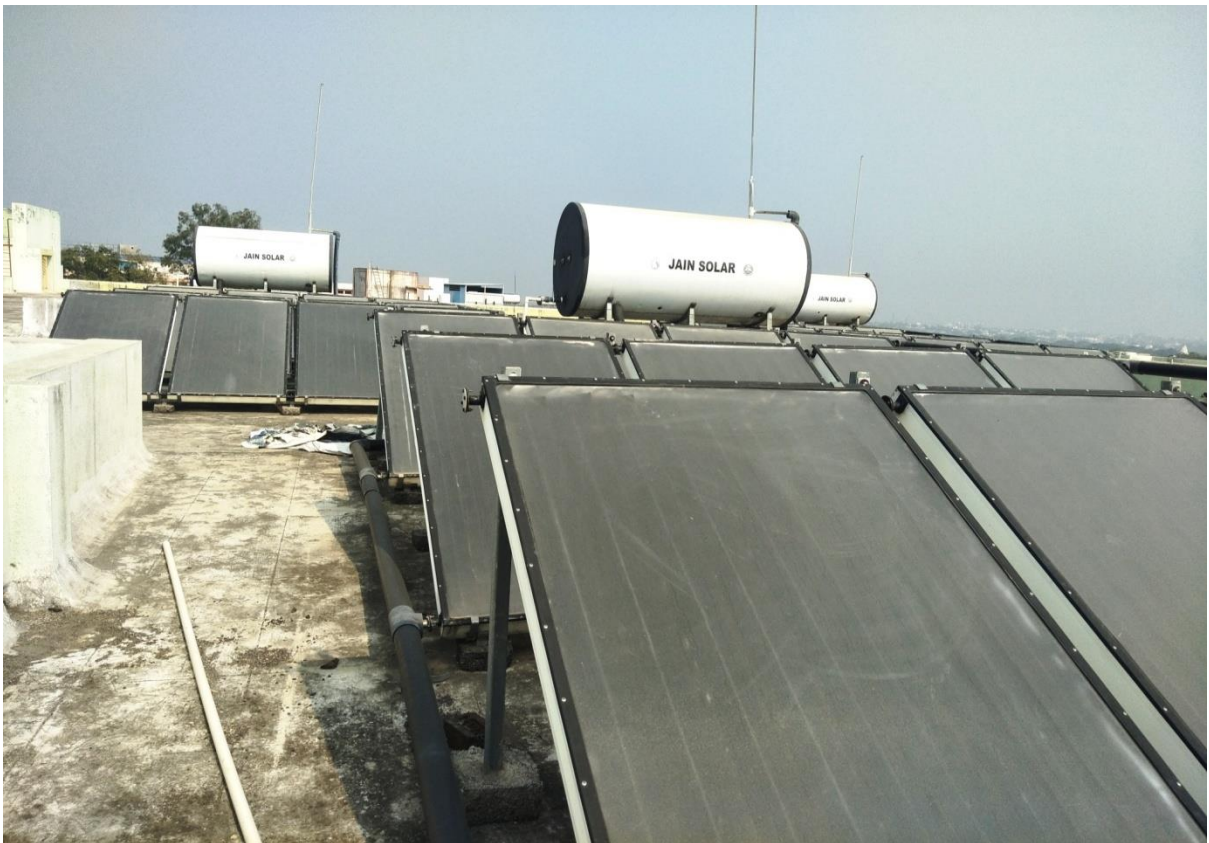
Fig . No.2 Solar Water Heater at Hostels' Rooftop
