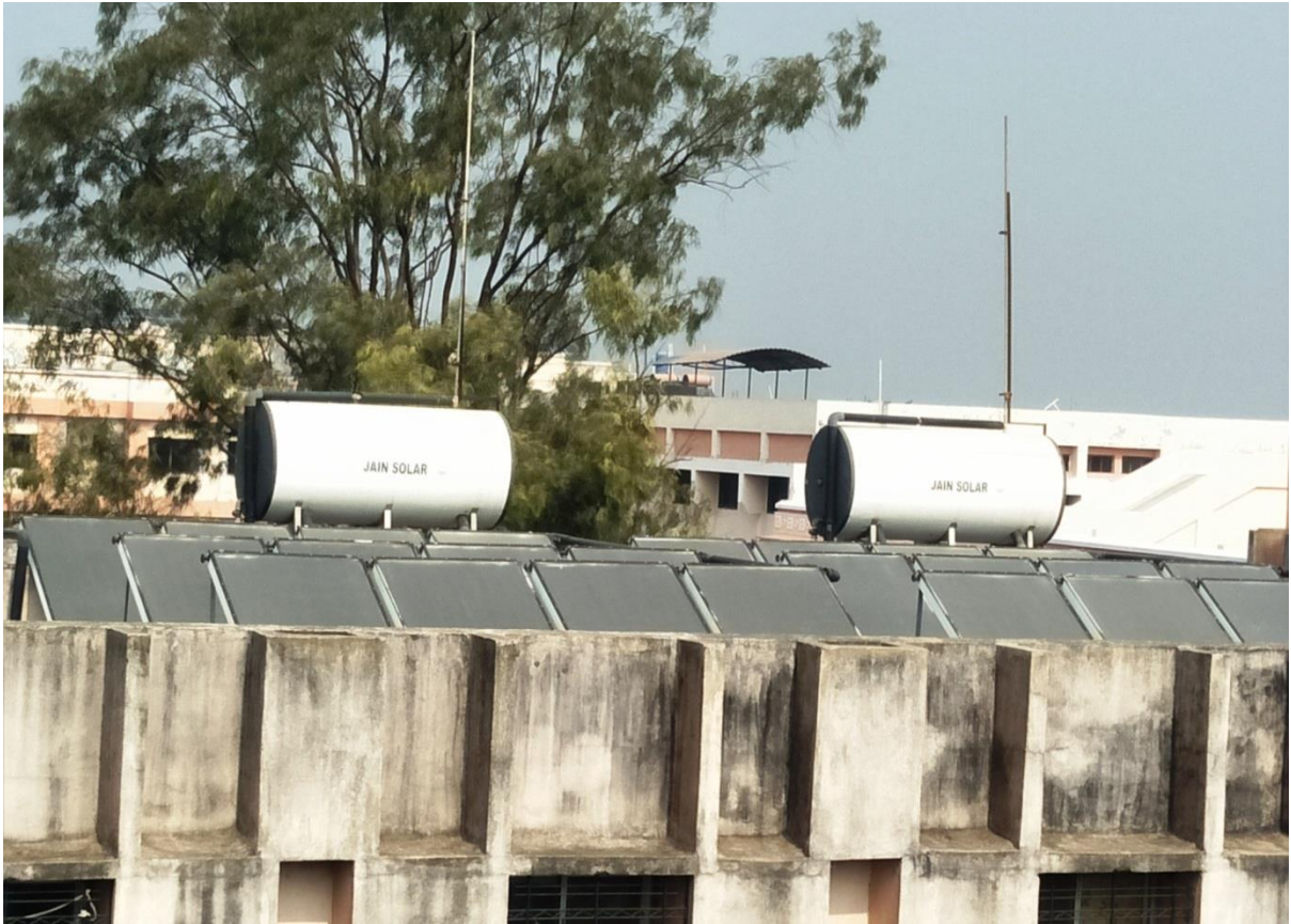
Fig . No. 1 Solar Water Heater at Hostels' Rooftop
