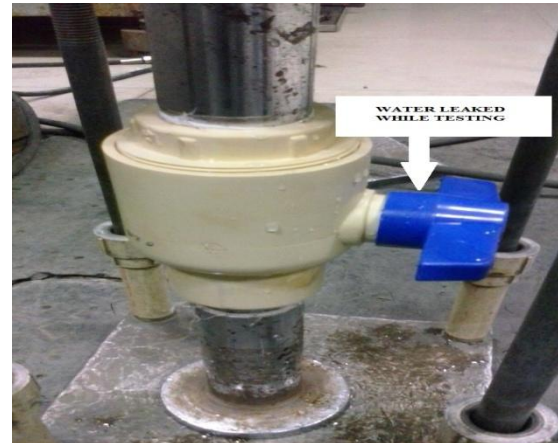
Figure 4. Ball Valve leaked from its spindle
